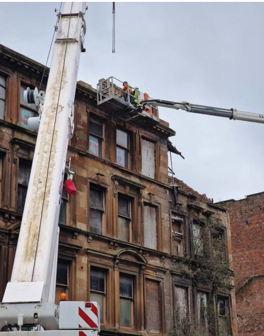
Demolition of the C-listed India Buildings has cost £1m (Image courtesy of Paul Sweeney)
