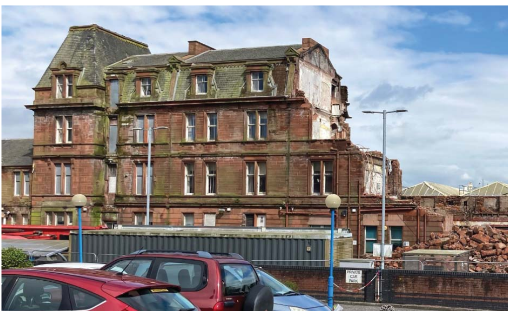
A surviving section of the north wing on 29th May 2024, as substantial demolition works to the tower and north wing neared completion (Credit: SAVE Britain's Heritage)
