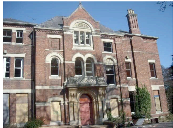
Copsewood Grange, deteriorating despite a planning condition to retain the building.
