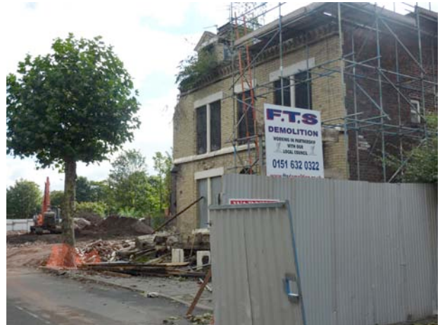
Shameful: fine Victorian houses in Ducie Street, Granby, Liverpool, under demolition in November 2010. Despite the axing of HMR funding the council seems intent on continuing Pathfinder clearances.
