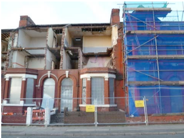
SAVE's landmark judgment means that Pathfinder demolitions will face tighter controls and be subject to closer scrutiny
