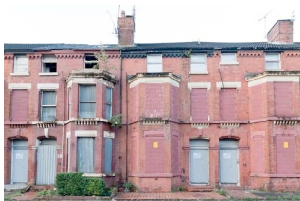
These houses in Kelvin Grove, Liverpool, were in near perfect condition before being emptied, tinned up and left to rot using HMR funding. Photo: Mark Loudon
